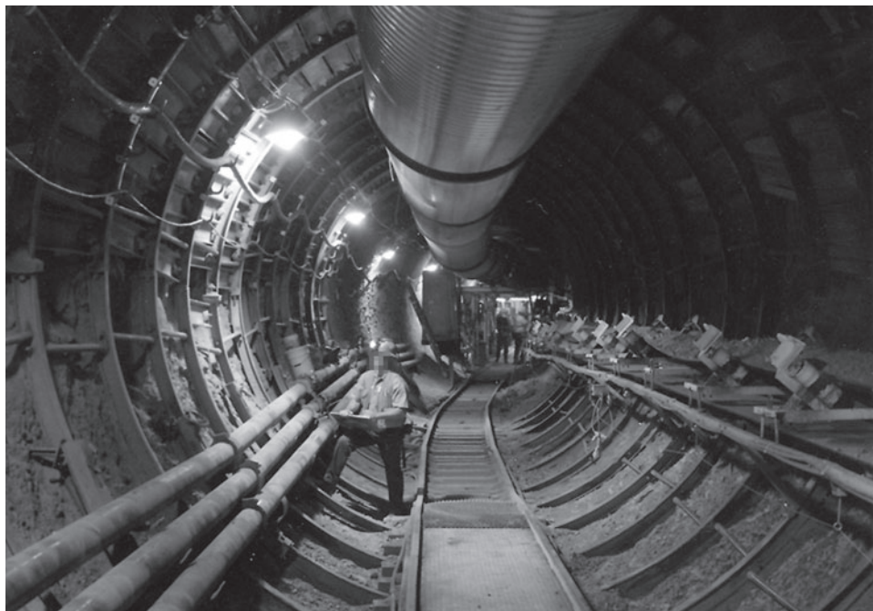
Figure 2: The 1.7-Mile Tunnel Built for Scientific Studies near the Potential Repository Area
